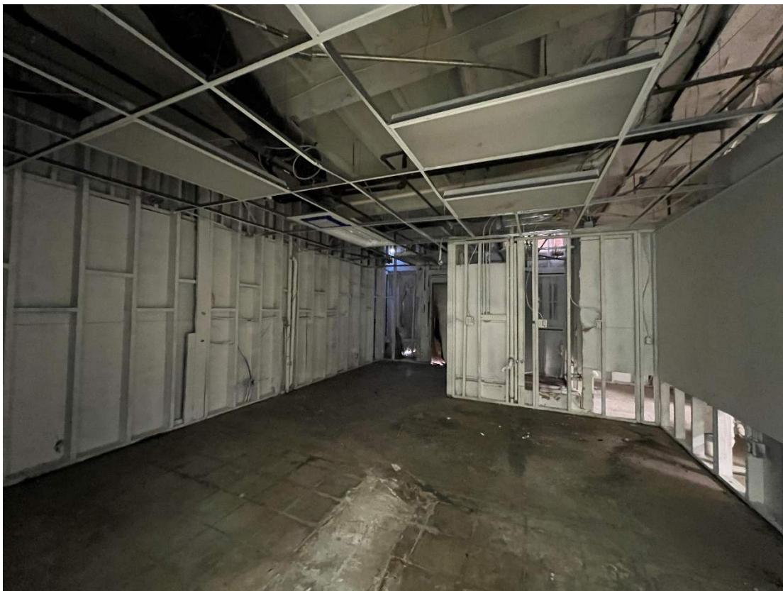
Fire Damaged Office
