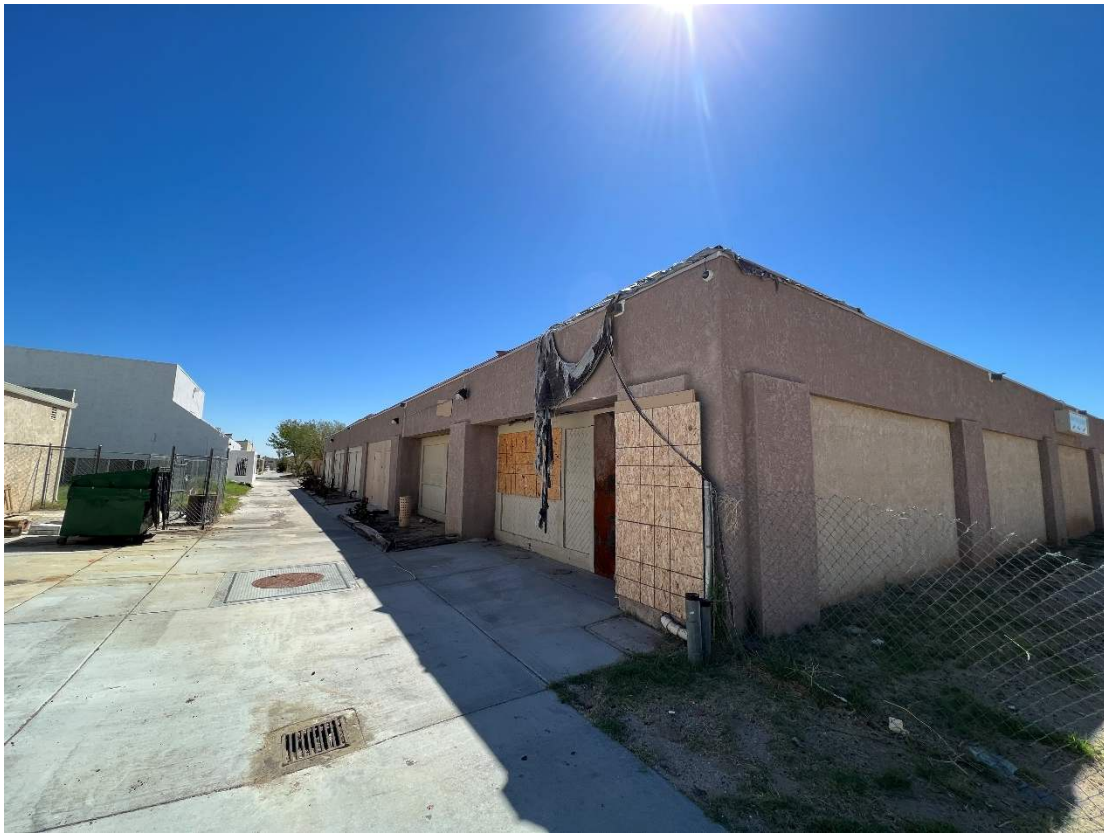
View along North Alleyway at Fire Damage Area
