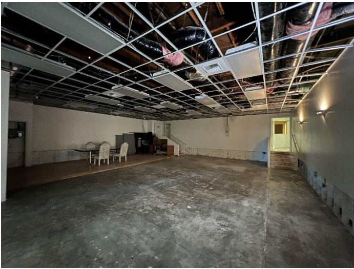
Fire Damage Area
